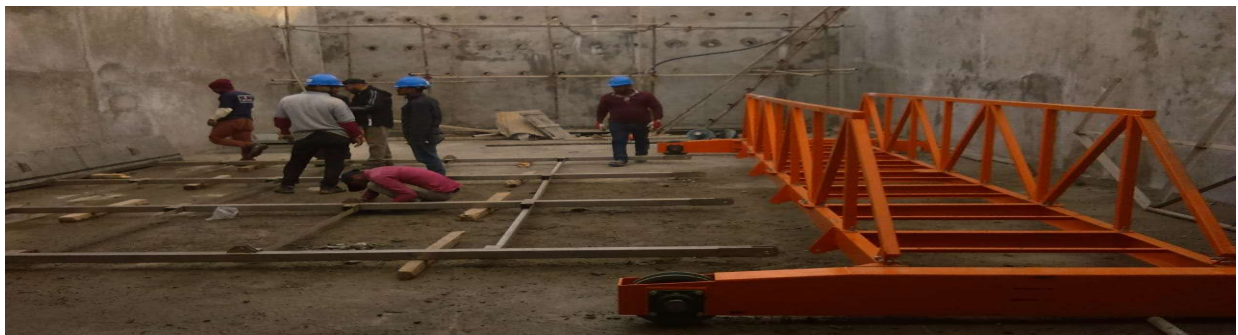
Design, Engineering and Manufacturing of 1.4 MGD Water Treatment in Filtration plant , Nilore Islamabad ,2019
