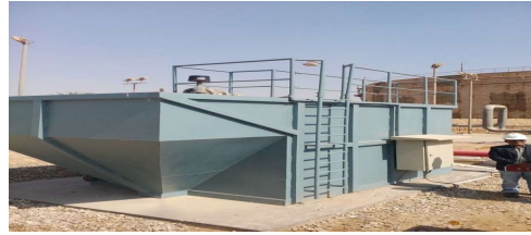
Extended Aeration STP, Asian petroleum
