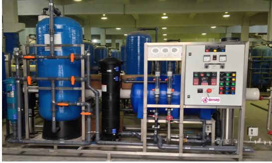
RO package plant, Lebanon FZ industrial area
