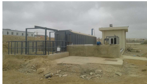
Package SBR unit , HUB
