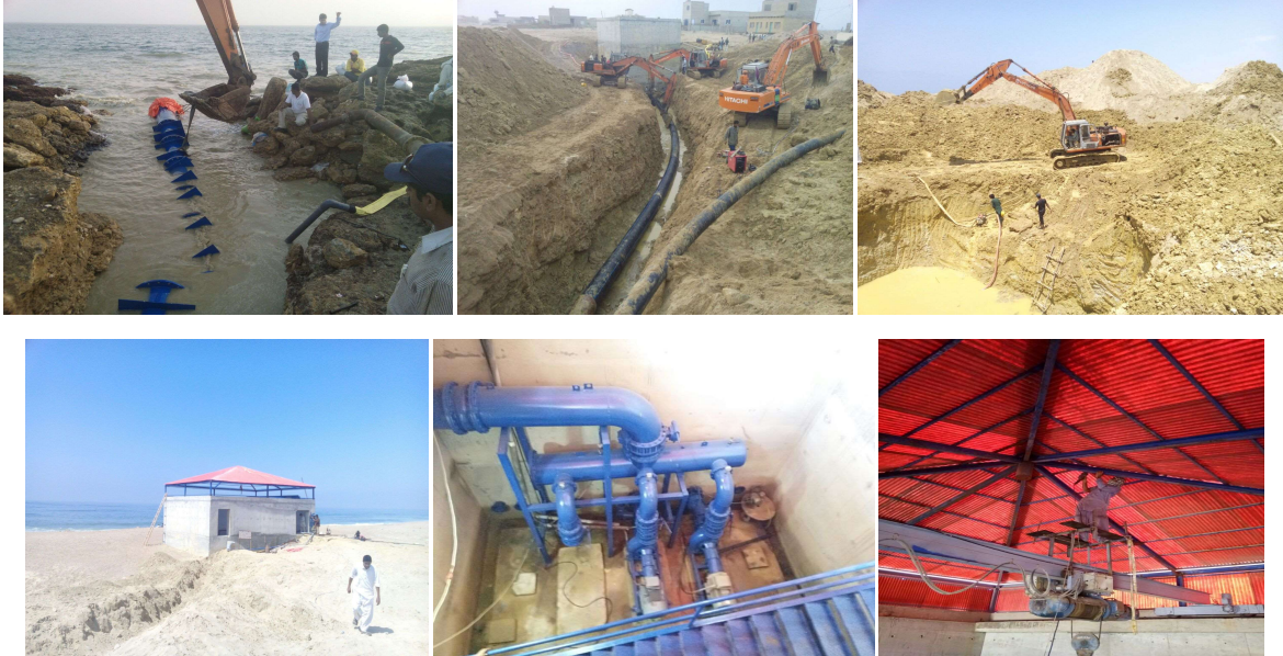
Design and Engineering of 14 MGD Sea Water Intake and pumping station at Karachi , Hawaks bay, Pakistan 2015
