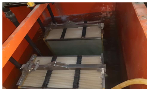
MBR effluent treatment unit, Karachi
