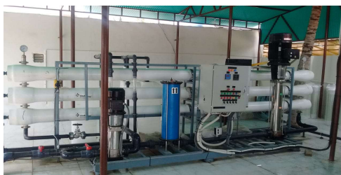
Skid mounted RO package units, Iran
